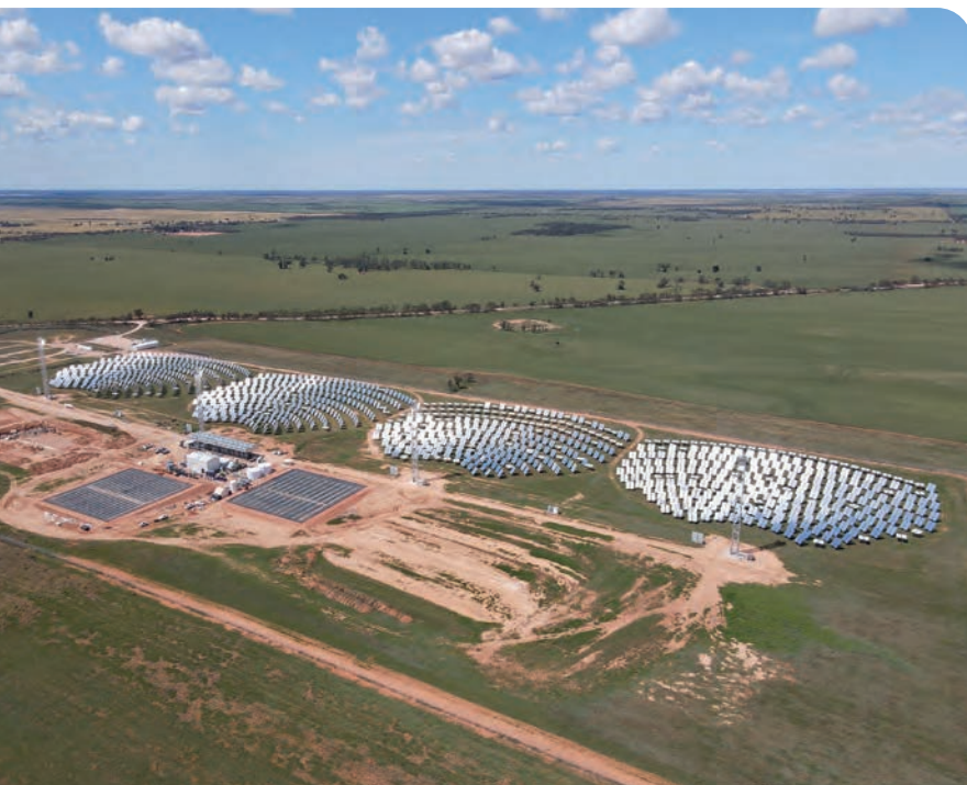
► Figure 4. Four RayGen solar towers during commissioning. RayGen's storage construction is nearing completion and will be operating commercially in early 2023.
